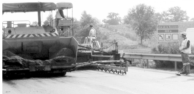
Figure 1. Research personnel of the BG BAU accompany the construction of Warm Mix Asphalt on A 81 near Laval in France.
