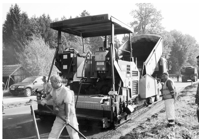
Figure 2. Installation of Warm Mix Asphalt in close proximity to Ljubljana in Slovenia.
